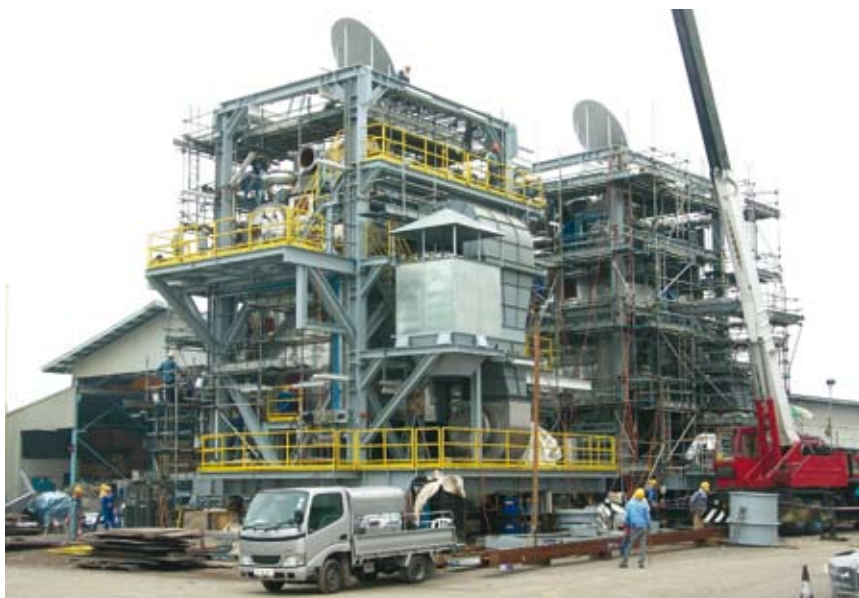
The two boiler plant skids for Prosafe's "FPSO UMUROA"
