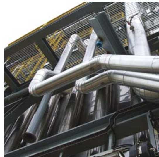
The piping arrangement is part of Aalborg Industries' supply
