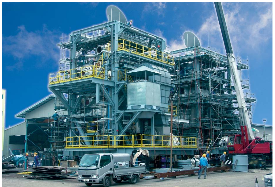
The two boiler plant skids for Prosafe's "FPSO UMUROA"
